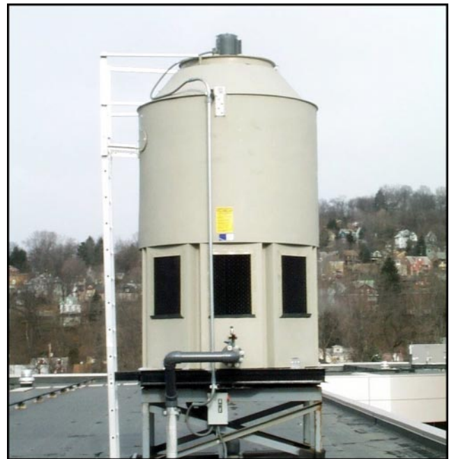
Built-in pockets reinforce the tower bottom so that the tower can be easily mounted on standard I-beams or imperfect pads. A plastic cooling tower used at the Conair plastics processing plant in Pittsburg, Pennsylvania.
