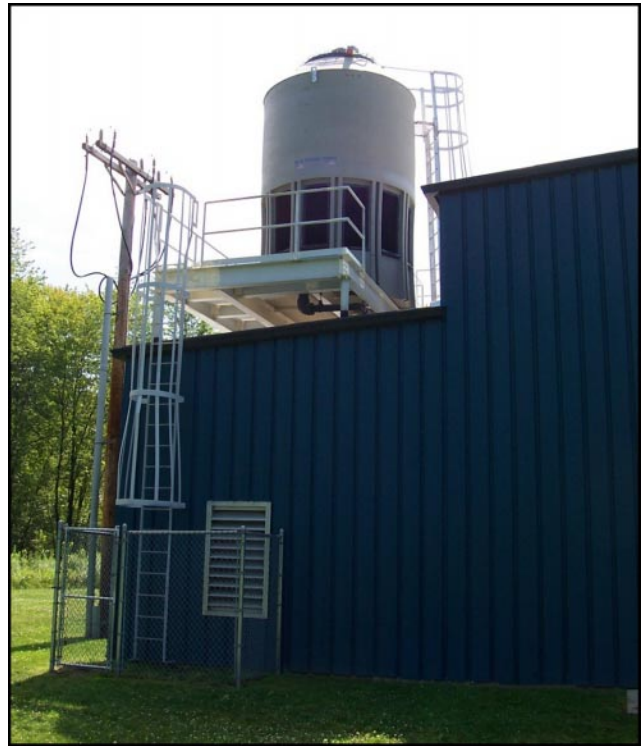
Plastics' lighter weight makes it easier to place cooling towers on top of structures. A plastic cooling tower used for a forging application at Meadville Forging, Meadville, Pennsylvania.
