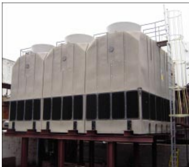
Modularized engineered-plastic tower arrays increase cooling capacity up to 2,000 tons. An engineered-plastic cooling tower installed at Elan Chemical in Newark, New Jersey.
