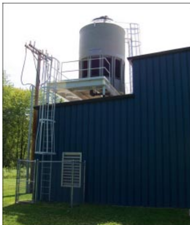
Engineered-plastics' lighter weight makes it easier to place cooling towers on top of structures. An engineered-plastic cooling tower used for a forging application at Meadville Forging, Meadville, Pennsylvania.
