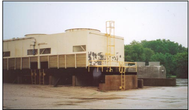
Old metal cooling towers are a classic “money pit” for plant maintenance personnel that rely on cooling towers to support key process equipment.
