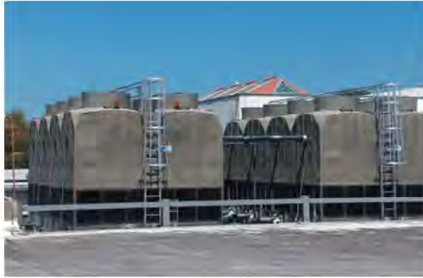
ALL IMAGES COURTESY OF DELTA COOLING TOWERS.
