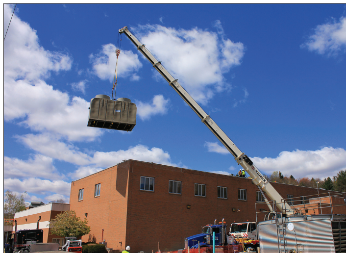
A crane lifts an HDPE cooling tower shell into place for installation.
