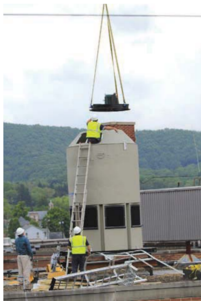
A Delta Paragon cooling tower is installed on the roof of Davis Memorial Hospital.
